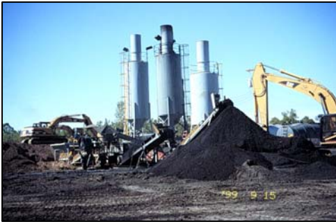
Figure 7-1. Ex-Situ Treatment at ACW
