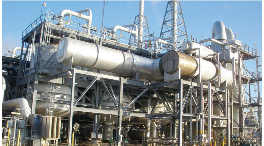
Flameless oxidizer system at a petrochemical plant.
